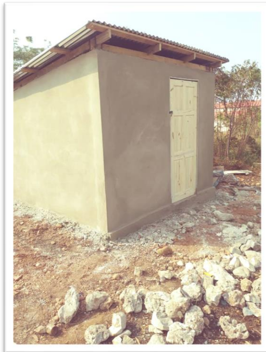
Feed storage unit
